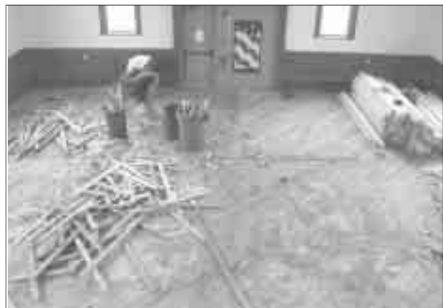
The crew from Danaher Custom Services removes the 1901 flooring from the main hall of Town Hall, to reveal the original sub-floor and 106 years worth of dirt. PHOTO BY JEANNE WILSON
